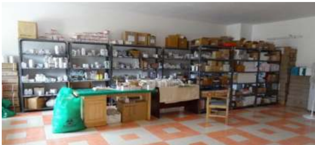
Figure 41. Unanchored racks with unrestrained medicines in inpatient pharmacy, top level of Service Block
