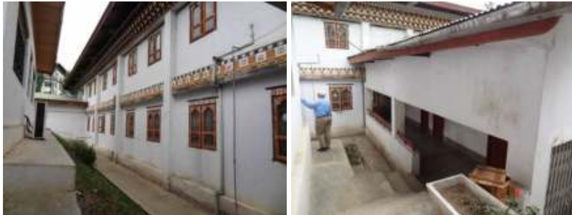
Figure 14. Views of back side of main community health buildings showing complex configuration
