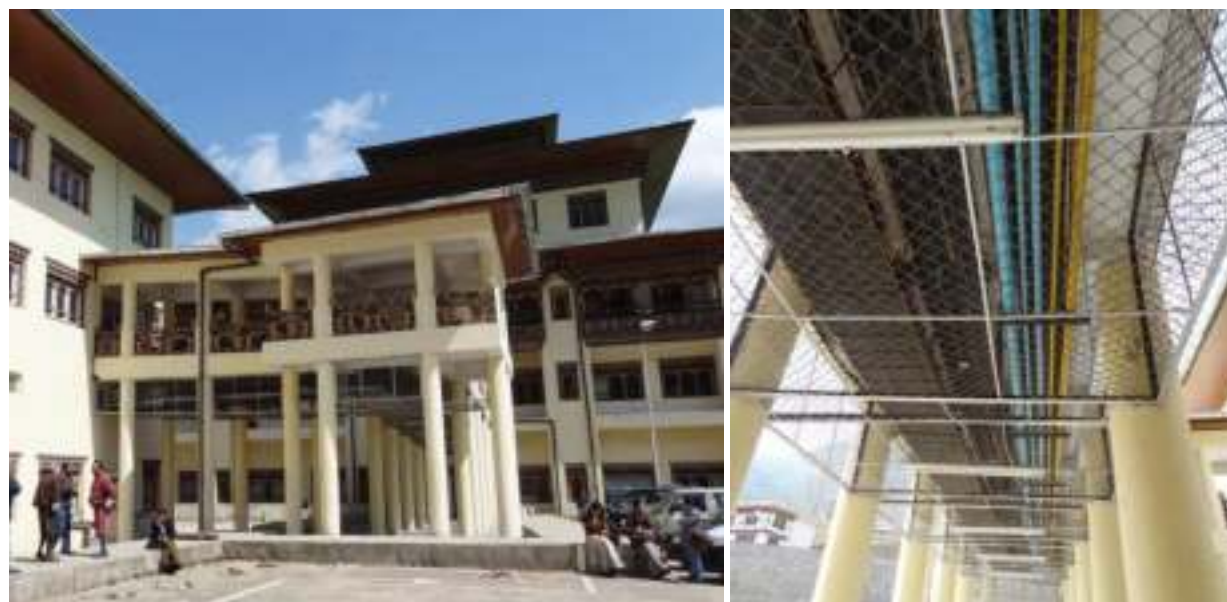
Figure 9. Bridge connecting Service Block to main hospital building (left); conduits and pipes suspended from walkway (right)
