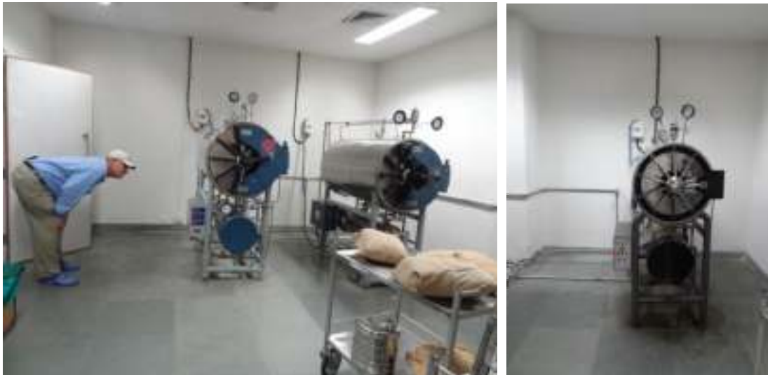
Figure 39. Inspecting unanchored sterilizers in the Central Sterilization and Supply Department (CSSD)
