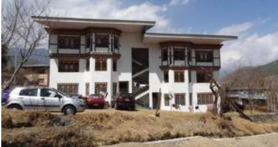
Figure 27. Nurses' quarters (Type 2) with 6 units and a large vertical discontinuity in the center of the building
