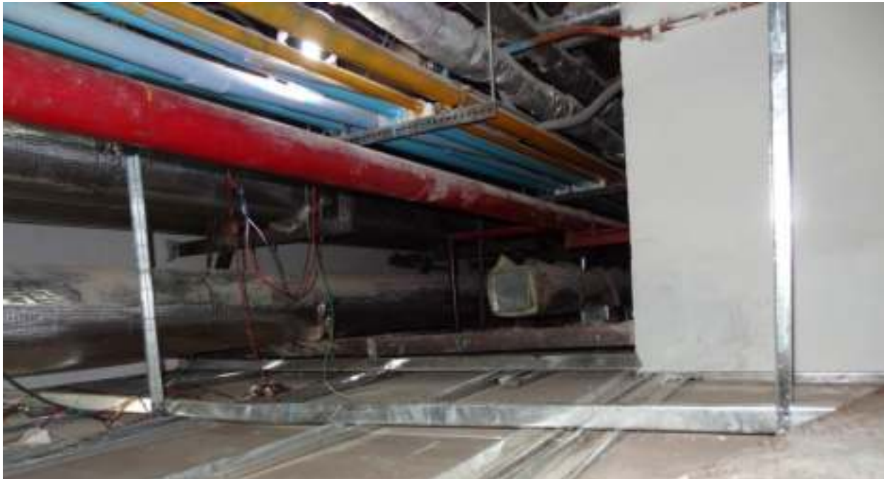
Figure 44. View above suspended ceiling showing support system and utility services. There is no lateral bracing for the suspended ceiling, fire and domestic water pipes, medical gas lines and steam pipes.
