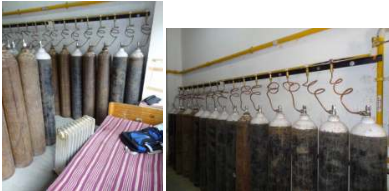
Figure 34. Unsecured medical gas cylinders; note the space heater
