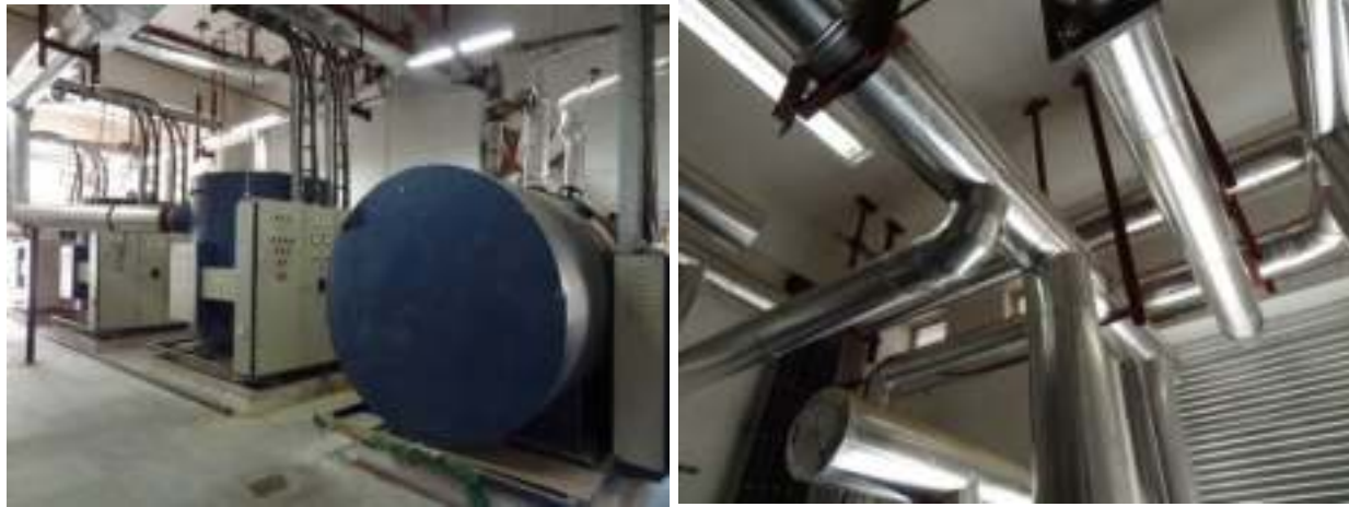
Figure 37. Unanchored boilers (left) and laterally unbraced pipes (right) in the Service Block
