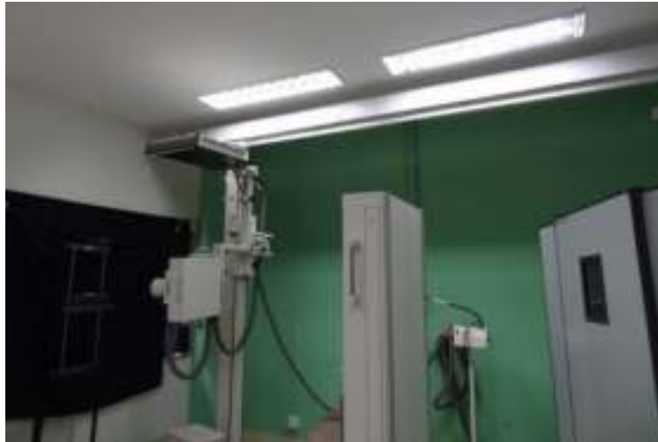
Figure 40. X-ray equipment supported by beam resting on seismically unstable brick partitions
