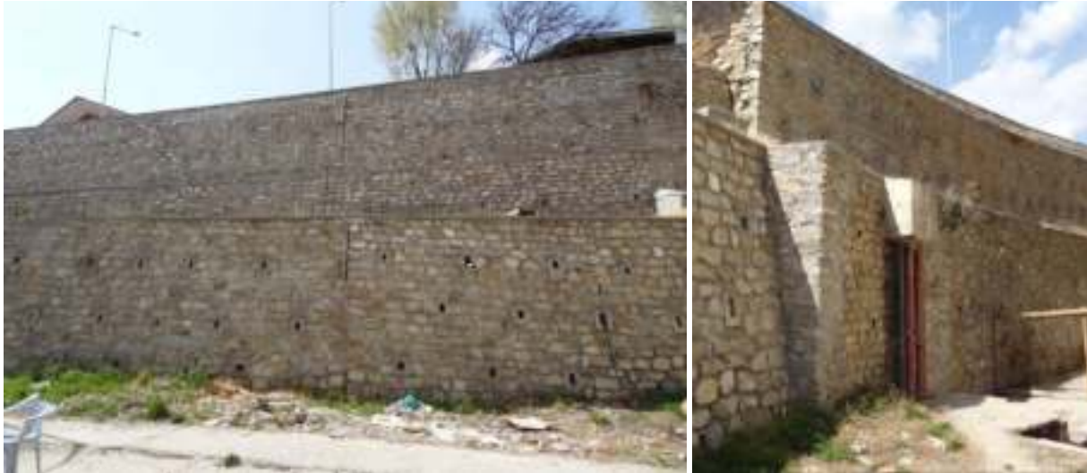
Figure 4. Retaining wall behind the Service Block (left); pipes emerging from the same retaining wall (right)
