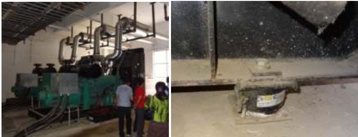
Figure 33. Unanchored emergency generator with inadequately braced exhaust system and unsecured batteries (left); non-seismic vibration isolators (right)
