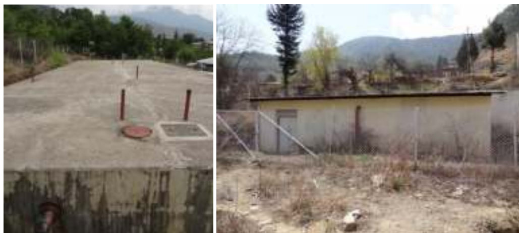
Figure 35. Drinking and fire suppression water storage tank (left); unreinforced masonry pump house below tank (right)
