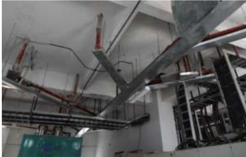
Figure 36. Suspended, unbraced wastewater pipes above a generator and electrical equipment in the Service Block
